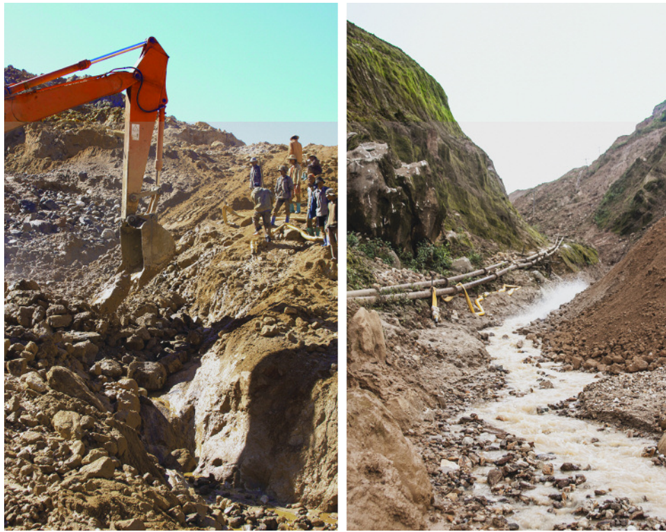
Figure 6. Left: Miners use excavators to remove gem-bearing overburden gravels. Right: The gravels are transported downstream to the washing plant using water supplied by the pipes. Photos by Hpone-Phyo Kan-Nyunt.
